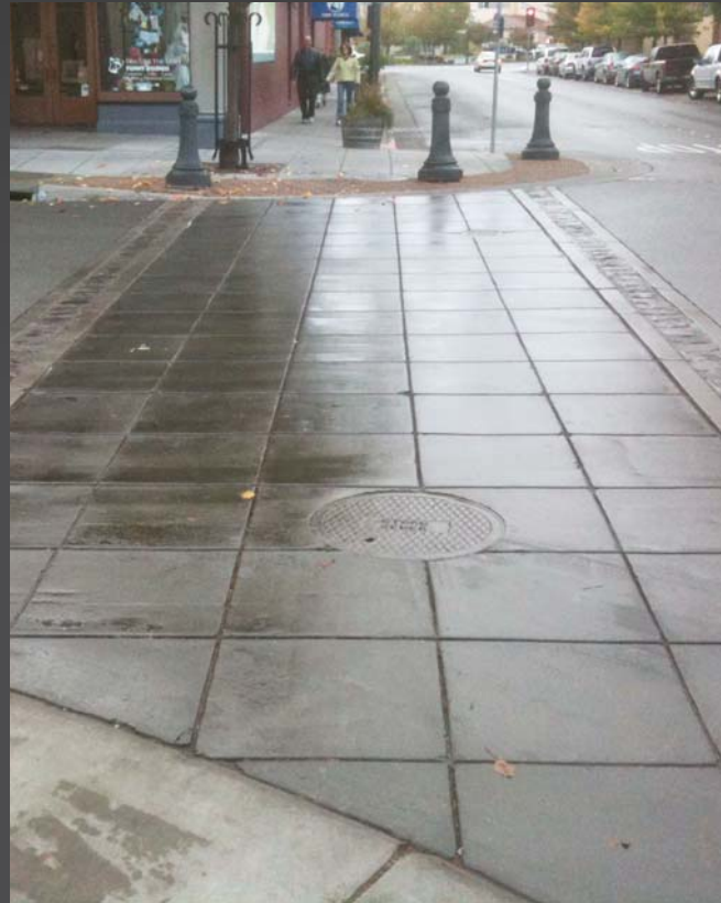
Scored concrete in crosswalk
